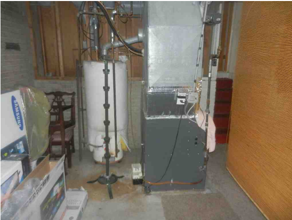
Furnace & water heater
