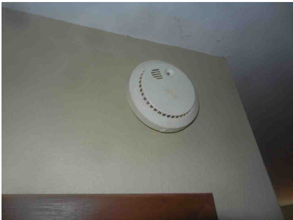
Smoke & CO detector
