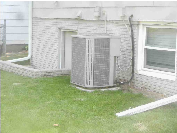
Central air unit
